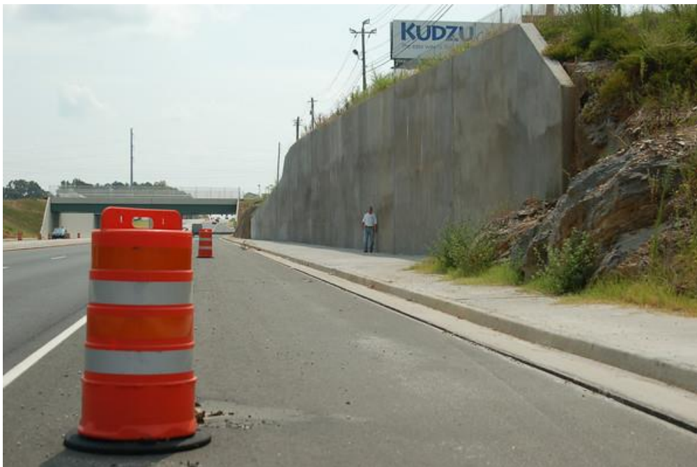
Figure 3 After view of Mercedes dealership from road showing client standing in front of 30 foot retaining wall, introduced to show change in visibility and access
